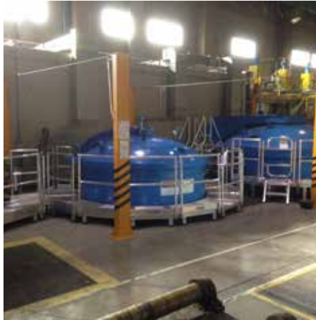
Walkway for Safe Access Around Industrial Inspection Hatches
